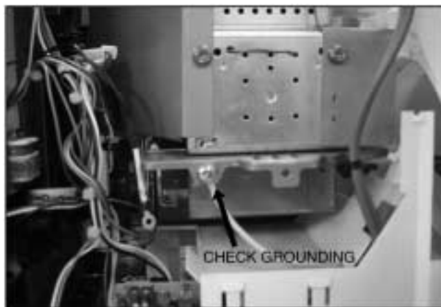
Grounding of the inverter circuit board
